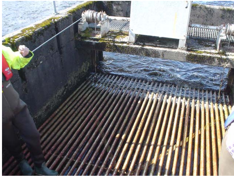
Figure 4.11: Bar screen raised above the water surface
