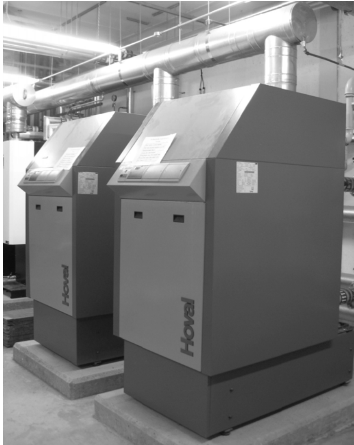
Figure 130: Building C: Boilers
