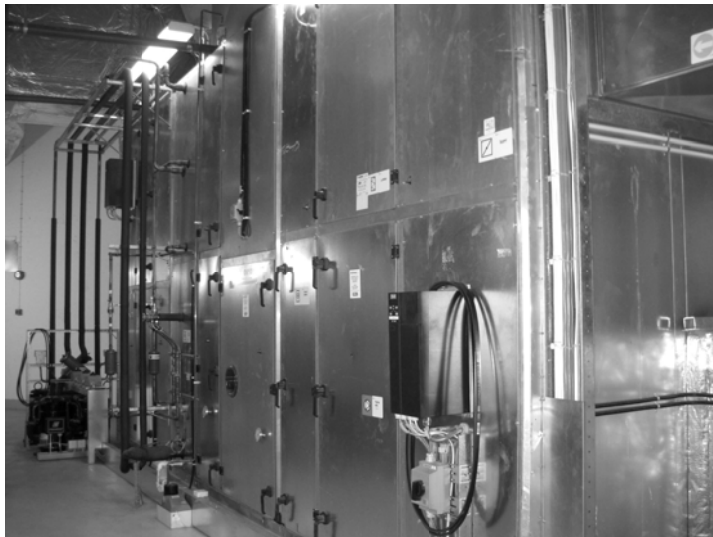
Figure 94: Building A: Air handling unit with heat recovery, located in the basement
