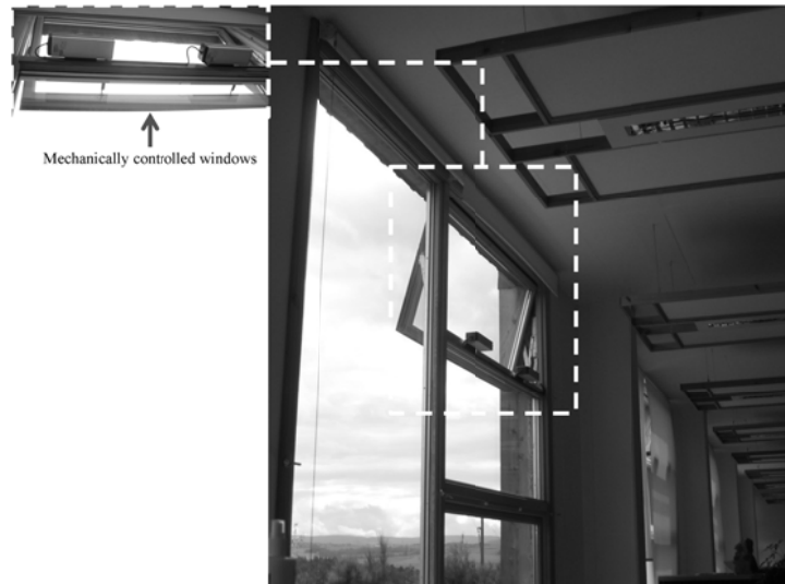
Figure 122: Building C: Mechanically controlled windows
