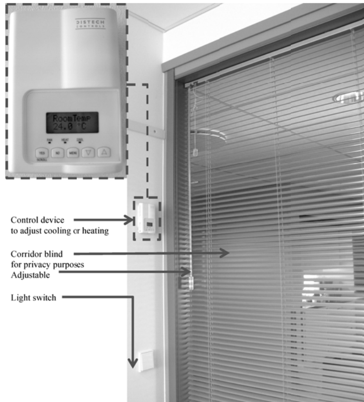
Figure 105: Building B: Control device, blind and light switch
