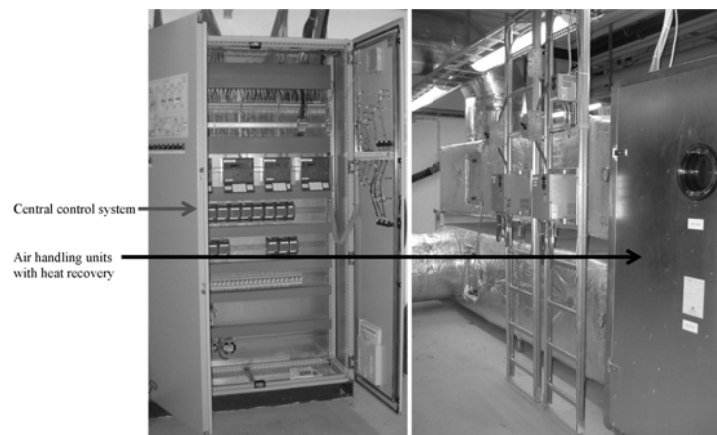
Figure 108: Building B: Air handling units and central control system
