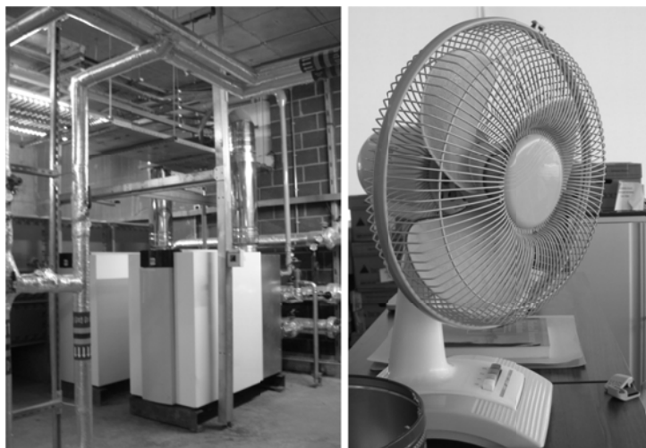
Figure 146: Building D: Boiler and personal fan as an adaptive opportunity provided based on occupants' request
