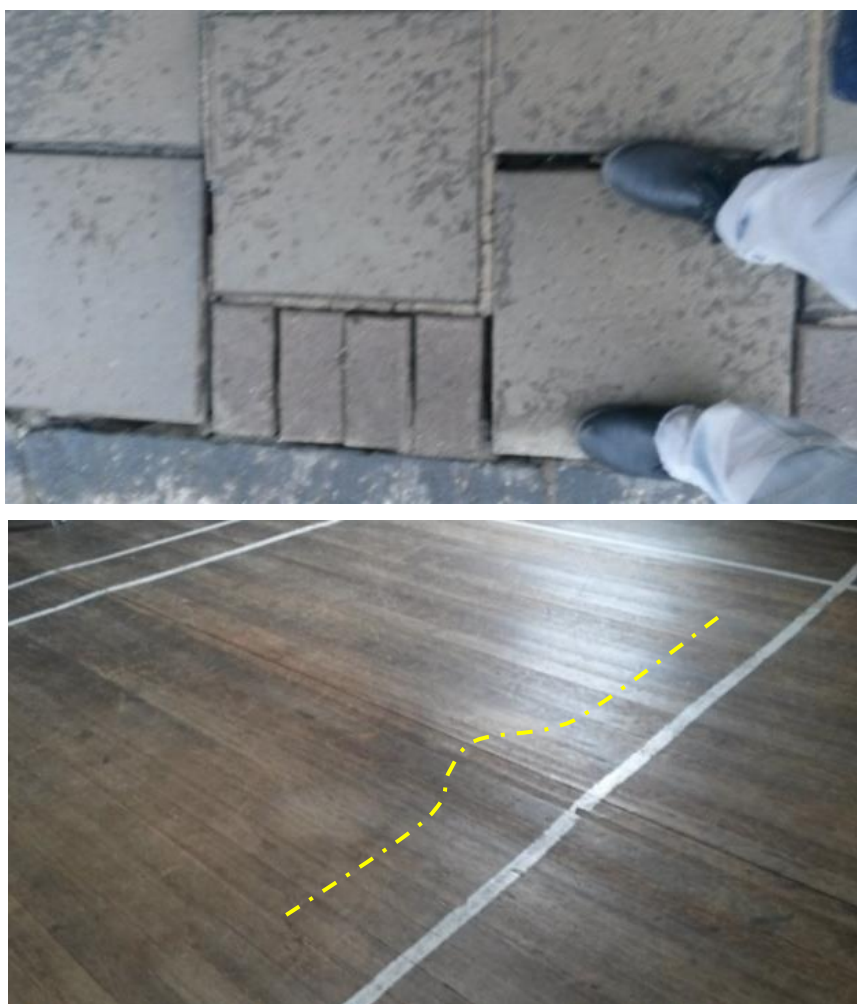
Figure 25: Irregular Cases of Faulty Floor: Bended Woods and Rocking Tiles (Said, 2014)
