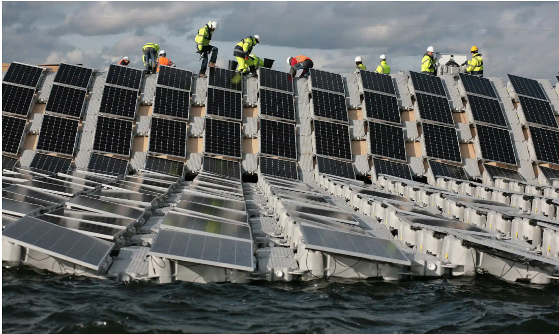
Figure 2.16: Modular Pontoon used at the UK's largest floating solar plant [52]
