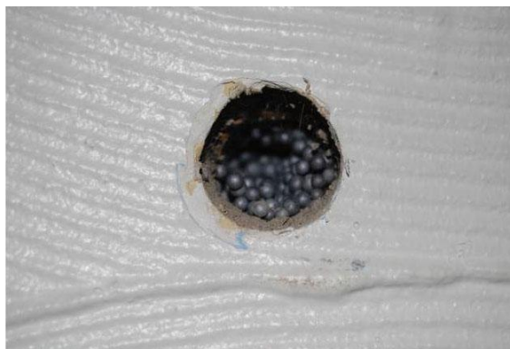
Figure 35 Polystyrene bead in void behind plaster
