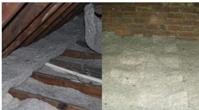
Figure 31 Loft insulation covering joists
