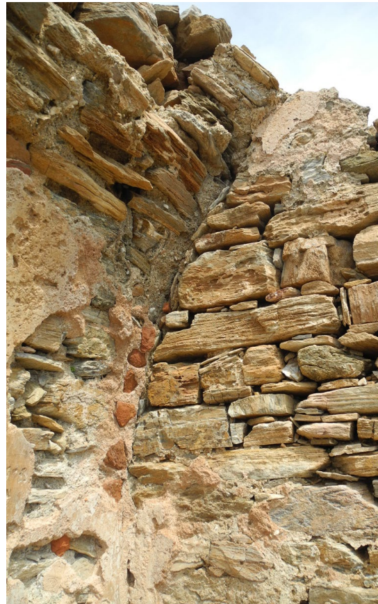
Fig. 131. Potsherds placed at the cistern's inner corners to reduce the risk of water leakage
