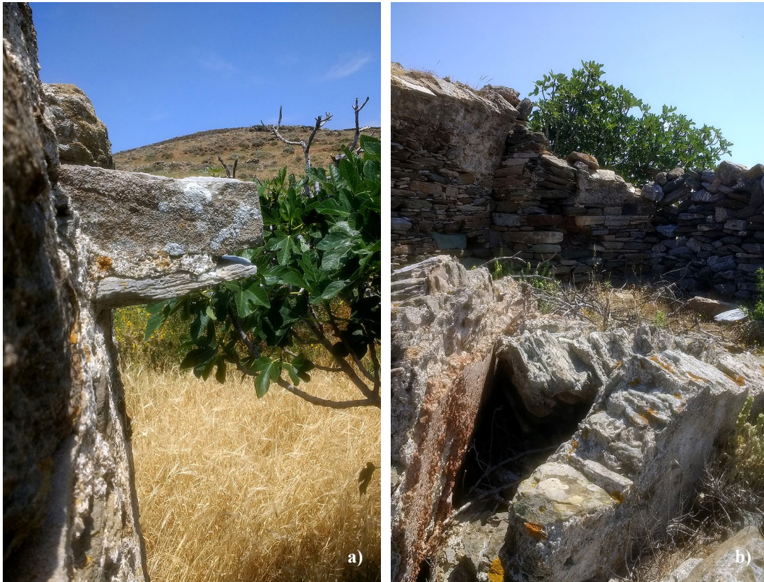
Fig. 75. Ch1 construction details: the waterspout (a) and the collapsed vault (b)
