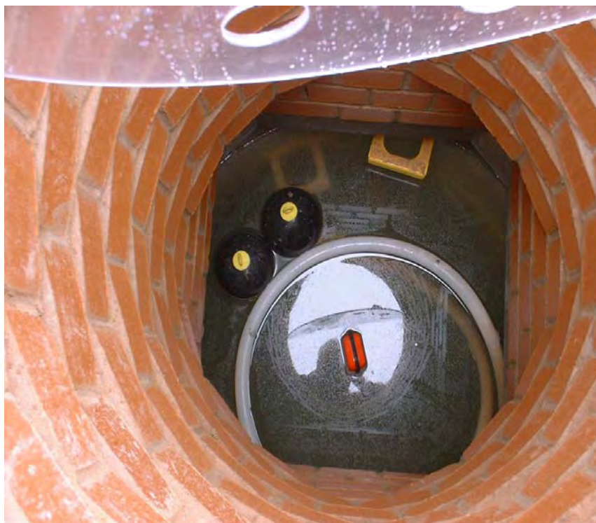
Figure 3-3 Collection chamber in tanked system provides sub-base water level control and appropriate maintenance (courtesy of Formpave Limited).
