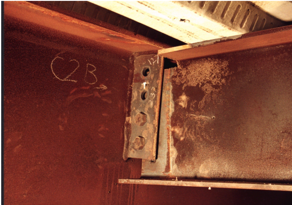
Figure 4.5: Connection failure in British Steel Test 2: Plane frame test
