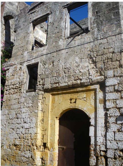
Figure 4: Deterioration of Rhodian sandstone and its architectural features
