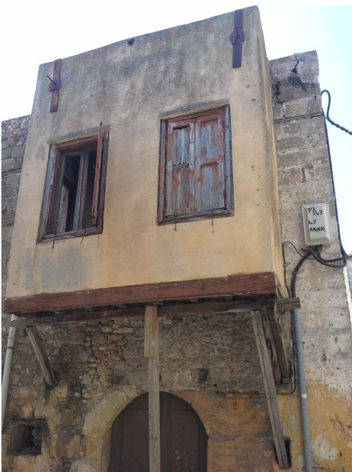
Figure 86: Voids in the structure due to the placement of sachnisi
