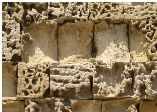
Figure 104: Deterioration of Globigerina Limestone
