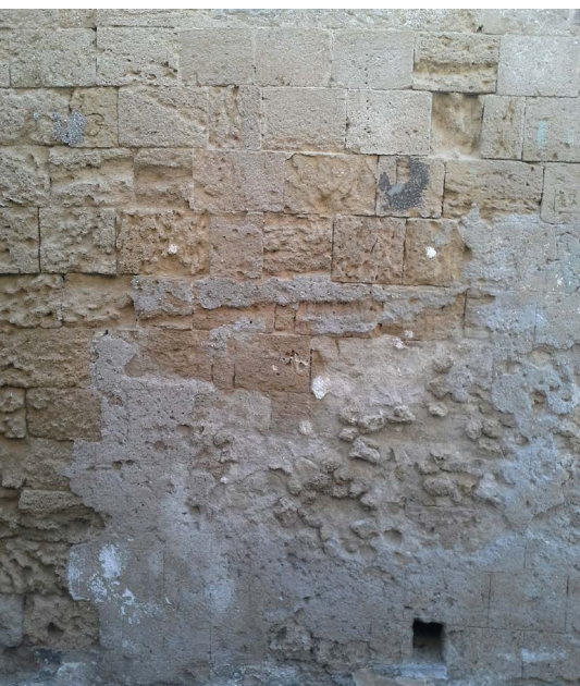
Figure 74: Use of cement for re-pointing and also for coating the surface of the facade
