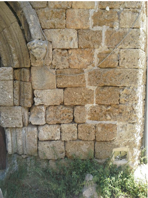
Figure 91: Biological growth and serious water absorption at capillary level
