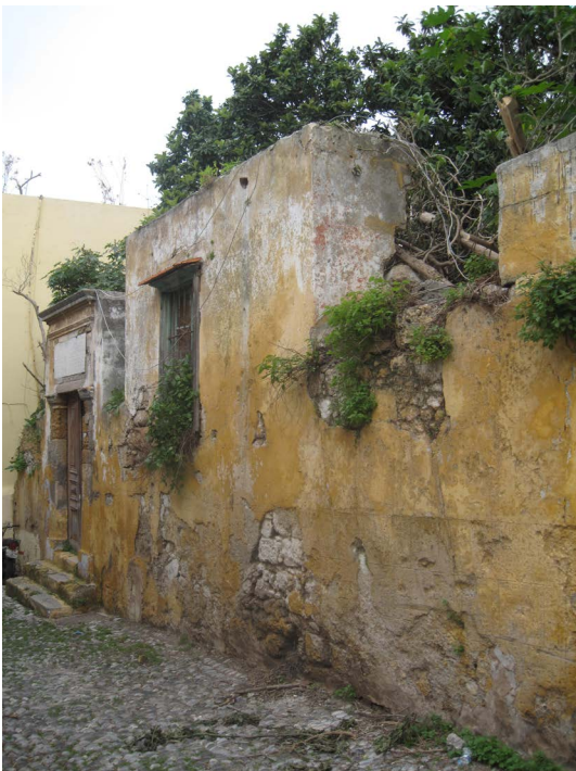
Figure 30: The abandonment and lack of maintenance exacerbate the decay of stone due to vegetative mechanisms
