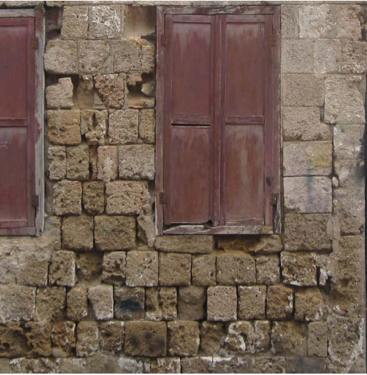
Figure 64: Loss of mortar on the joints and serious deterioration on the sandstone due to soluble salt
