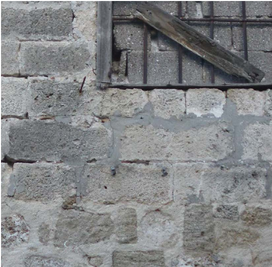
Figure 96: Hard cement mortar leading to moisture entrapment
