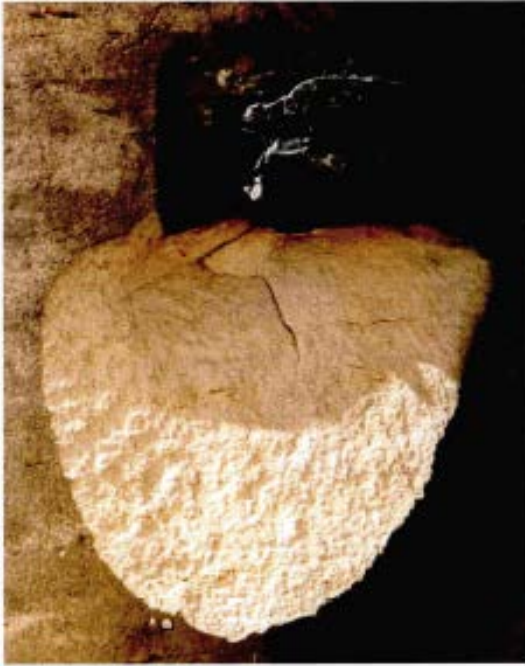
Figure 5: Decay due to mechanical damage leading to loss of compact material
