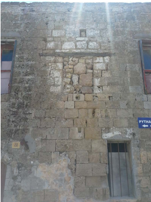
Figure 80: Blocked window on the facade filled with rubble and the decayed lintel of the window
