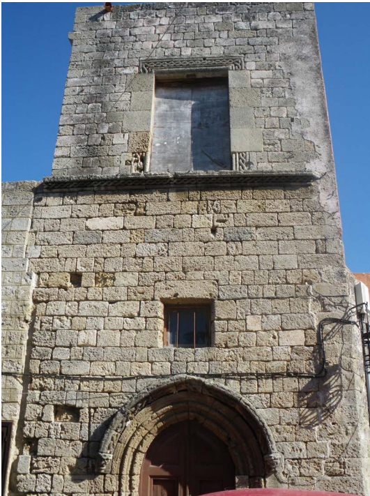
Figure 29: Dissolution of stone components due to salt erosion and transformation of \text{CaCO}_3
