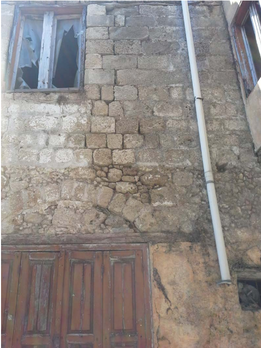
Figure 85: Arched doorway and loss of mortar in the joints
