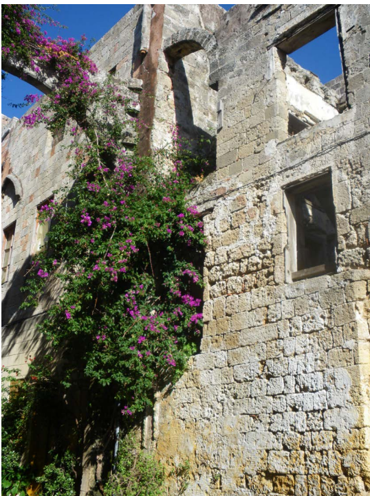
Figure 27: Biological colonisation and plants on the facade
