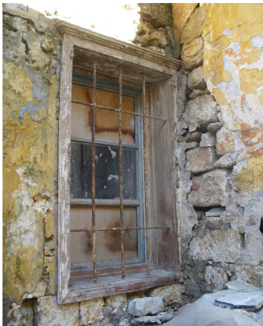
Figure 8: Disruption of the stone masonry near the windows from example in the Medieval Town of Rhodes
