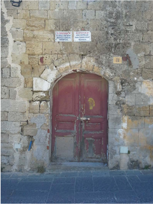
Figure 79: Deterioration of keystone of arched door and patina on the stone surface
