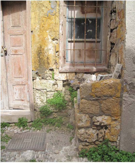
Figure 42: Biological growth in the stone masonry
