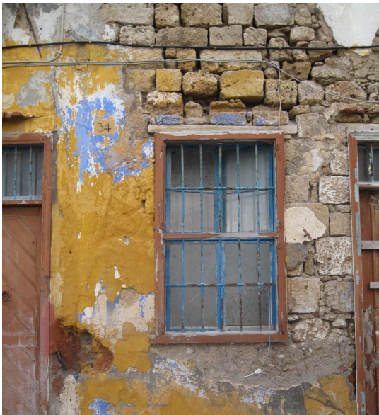
Figure 48: Disruption of the stone masonry due to salt erosion along with decay of mortar
