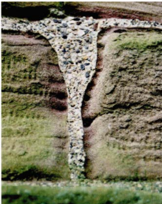
Figure 6: Hard mortar favours moisture entrapment in the sandstone rather than the mortar
