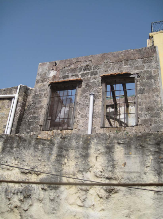
Figure 50: The roof in the back of the building has collapsed revealing 3 wooden beams
