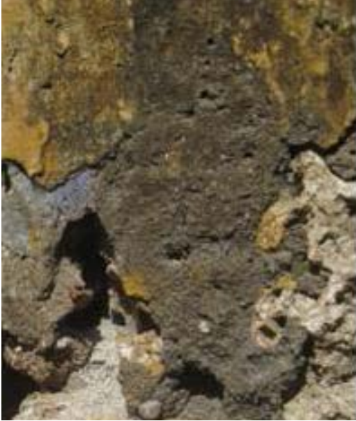
Figure 92: Granular disintegration of sandstone
