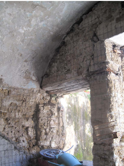
Figure 51: The extensive use of cement on the ground floor damaged irreversibly the structure of the masonry and the stone itself
