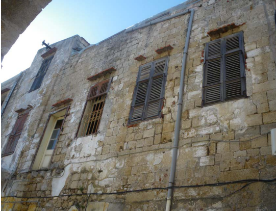
Figure 95: Loss of mortar in the joints
