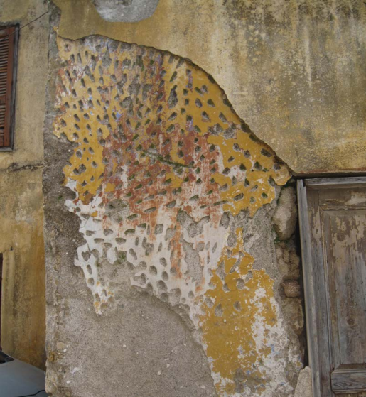
Figure 90: Loss of the last layer of coating and disruption of masonry at the windows edges
