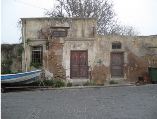
Figure 7: Hard mortar favours moisture entrapment in the sandstone rather than the mortar. Example from the Medieval Town of Rhodes
