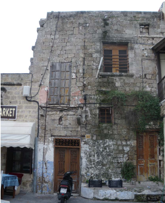
Figure 26: Salt erosion seen on the porous Rhodian sandstone together with structural cracks on the masonry
