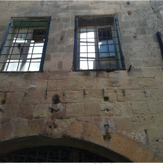
Figure 72: Deterioration of the keystone
