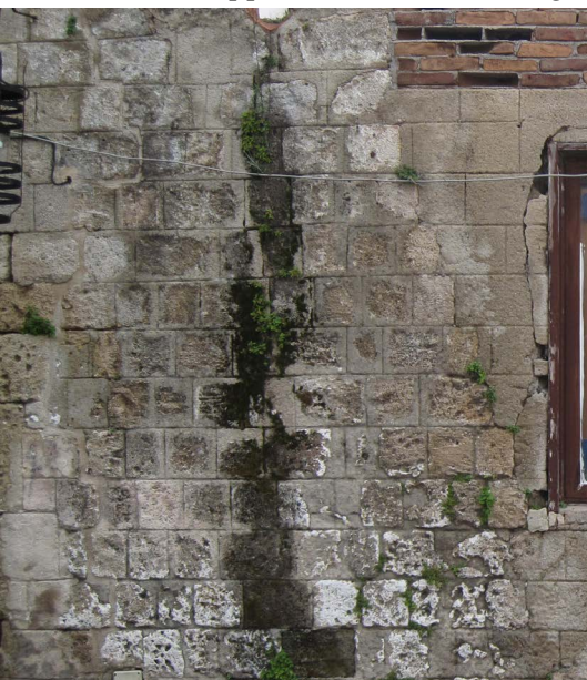
Figure 66: Salt efflorescence and black crust on the stone masonry due to poor rainwater goods
