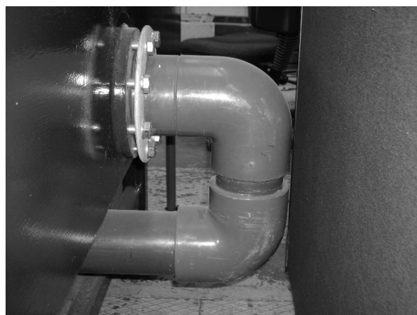
Figure 6.2: The inlet pipe to the flow-table tank
