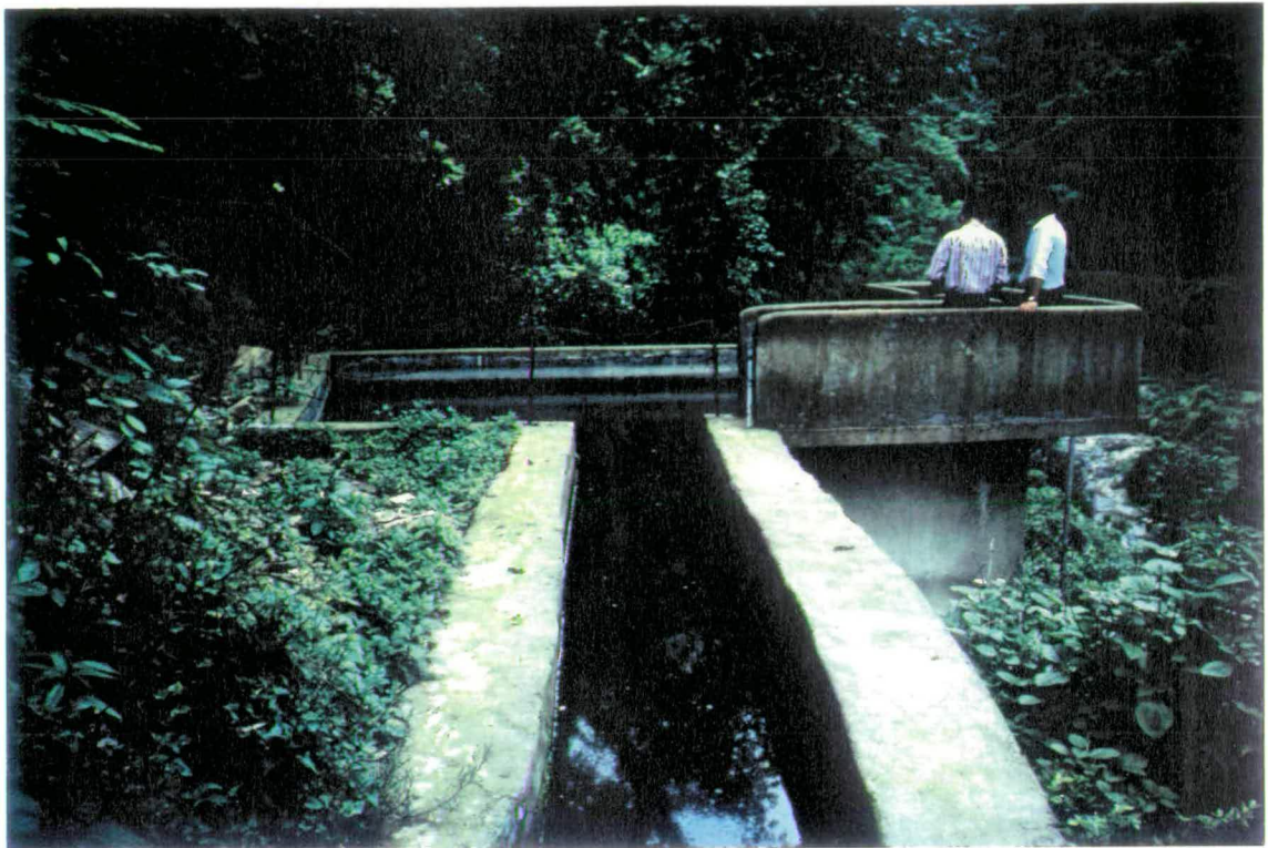
Photograph 5.14 Power channel and forebay for Bilkot 50kW project
