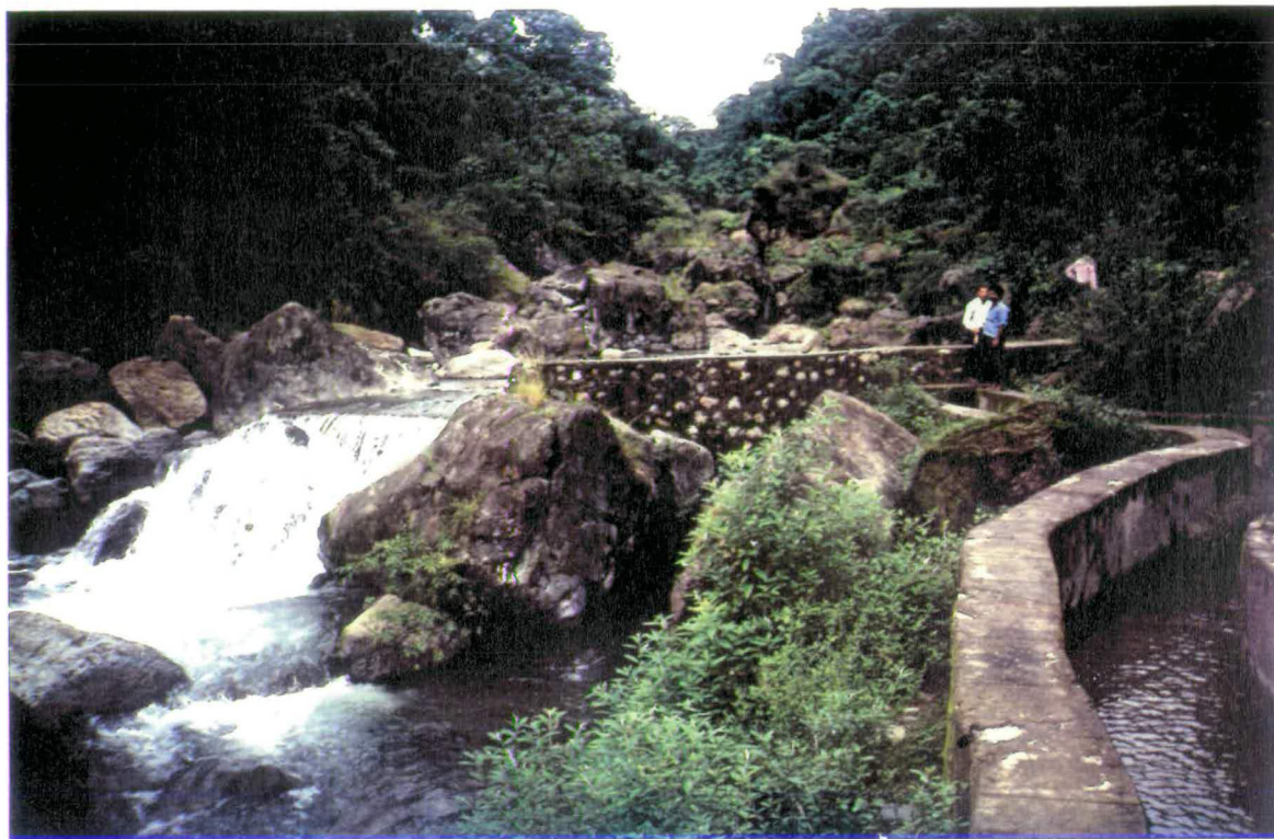
Photograph 5.17 Silted diversion structure at Kempti Falls MHP project
