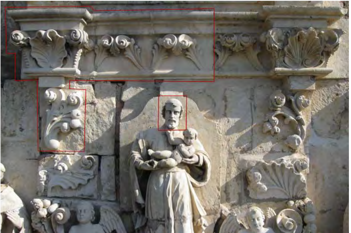
Figure 3.16 Detail of facade above window, showing inappropriate 1949 replacement carvings at left and central sections of cornice with original sections at right, as well as the 1949 replacement head of the central figure of St. Joseph. Note construction joints cleared of OPC mortar and awaiting new lime mortar. November 2010.
