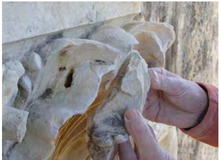
Figure 3.24 Pinning of detached drop pendant in zone C during Phase I in 2009.
