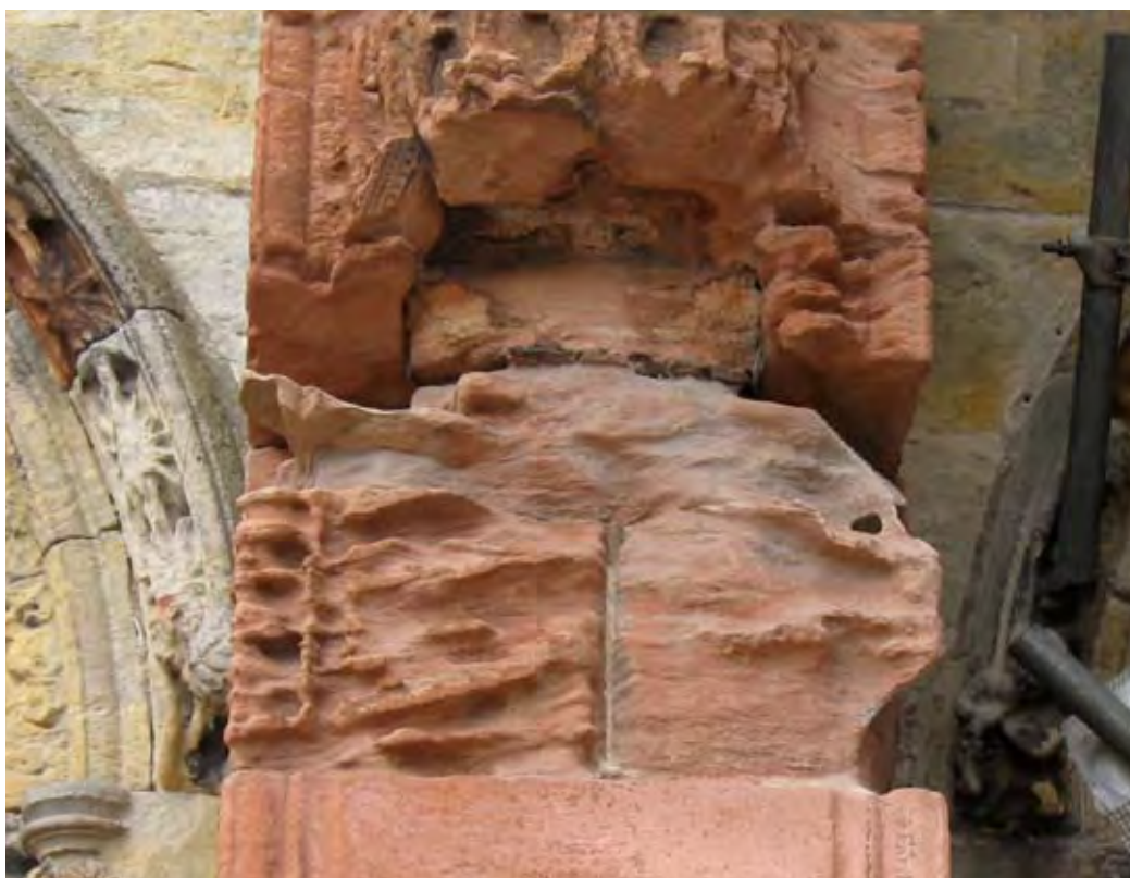
Figure 4.2 Severly weathered carved stonework on the south facade of Rosslyn Chapel. According to Boyes [Interview, 16 June 2011], the stonework will be stabilized with lime mortar at the open joints in order to prevent water ingress, however, no replacement of the carved stonework will be carried out as the stone is currently considered structurally stable.
