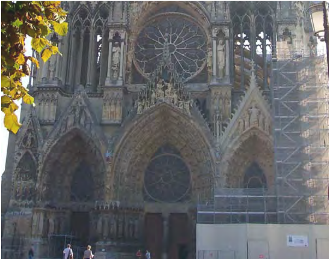
Figure 1.7 Reims Cathedral, France in 2004 during restoration and conservation work on the south portal.
