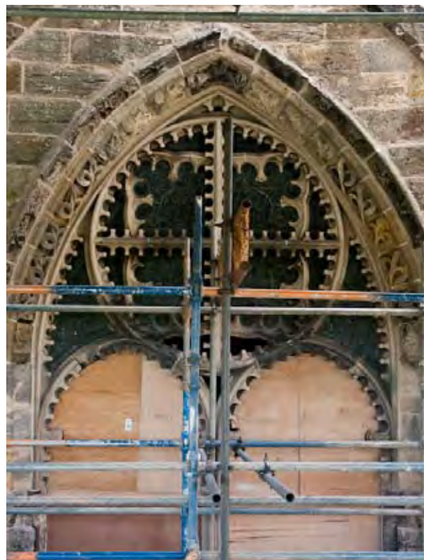
Figure 2.24 Great east window at Rosslyn Chapel in 2010 prior to replacement of section of tracery.
