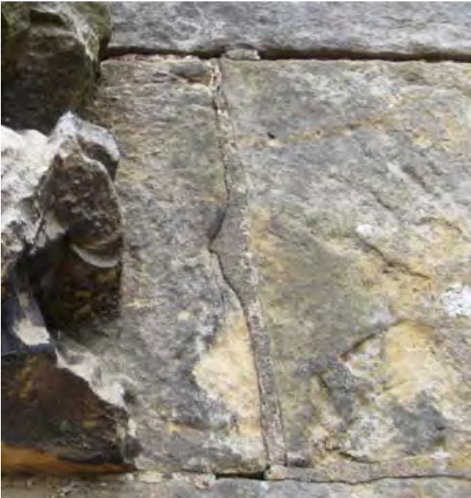
Figure 2.19 Examples of cement mortar that is causing preferential erosion of the adjacent stone surfaces.
