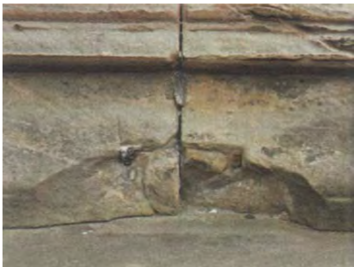
Figure 2.23 Damage to stonework at carved base course caused by oxide jacking of ferrous dog cramp.
