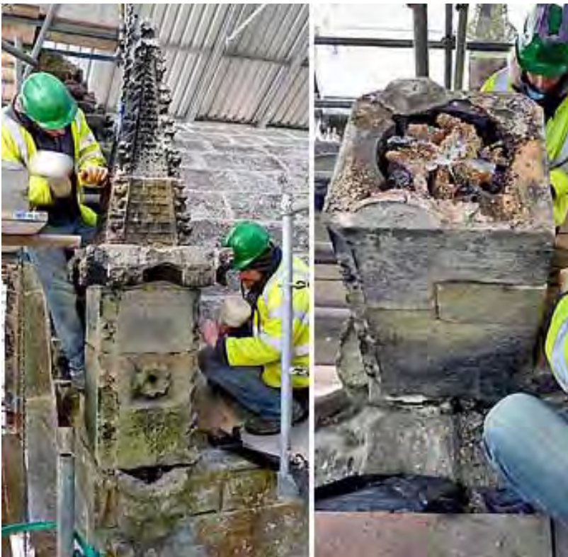
Figure 2.21 Deconstruction of N5 left side pinnacle during stabilization work in 2010 in order to properly re-bed and secure pinnacle.
