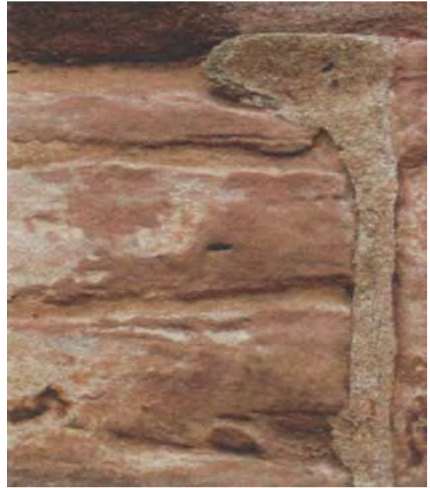
Figure 2.20 Detail of cement mortar on red sandstone surface that has caused significant preferential erosion of the stone.
