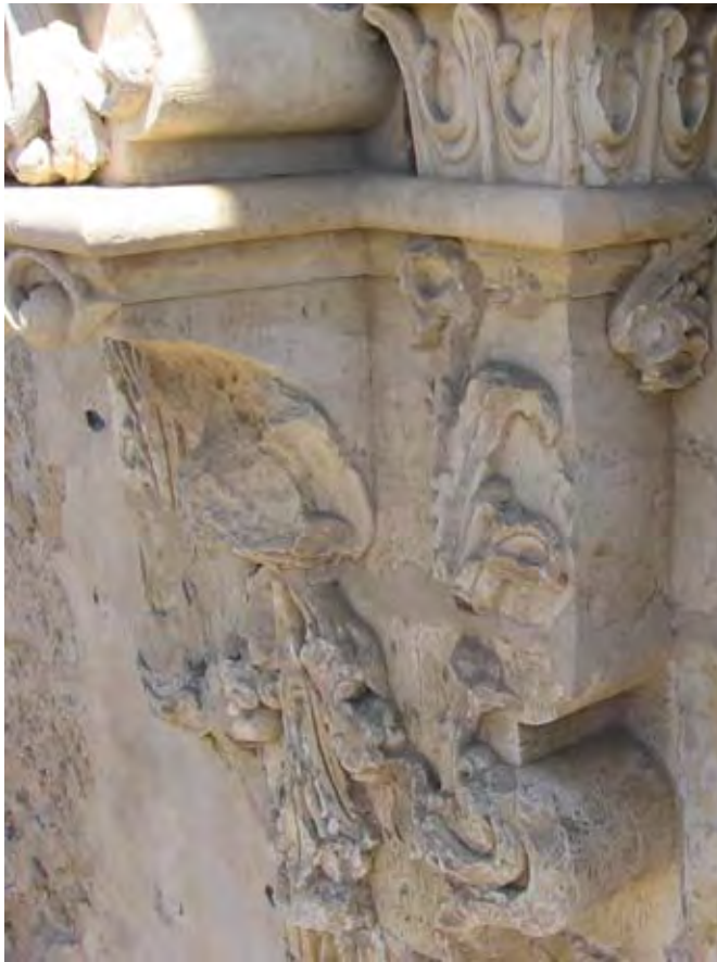
Figure 3.30 Detail of area below St. Joachim figure in Zone W, showing area of missing original carved stonework beneath pedestal. February 2009.
