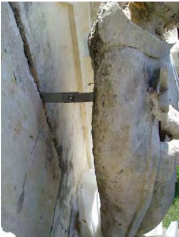
Figure 3.23 Stainless steel lateral tie-back installed to secure St Francis figure during Phase I in 2009.
