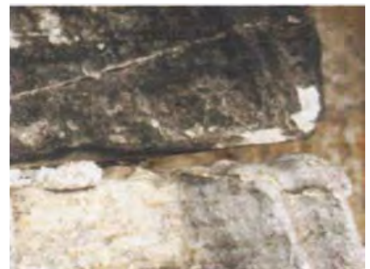
Figure 2.22 Detail of construction joint at buttress pinnacle showing loss of bedding mortar that has caused the stonework to become structurally unstable.
