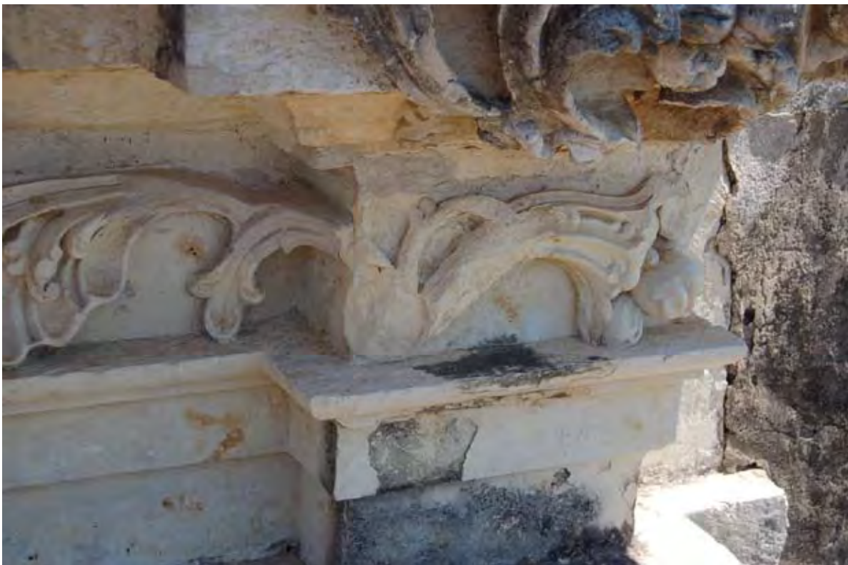
Figure 3.17 Detail of Zone C showing areas of cement mortar repairs and areas of heavy scaling, delamination and biological growth below the cornice, where stone tends to remain damp after periods of heavy rain. February 2009.
