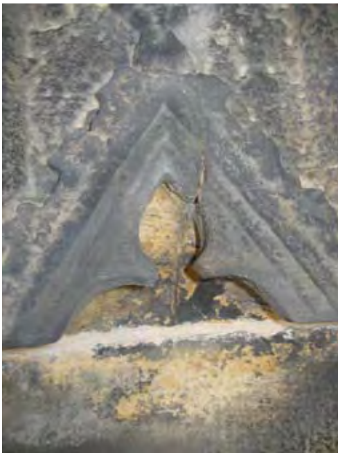
Figure 2.34 Crack along carved element on S5 pinnacle after being consolidated with acrylic resin. June 2011.
