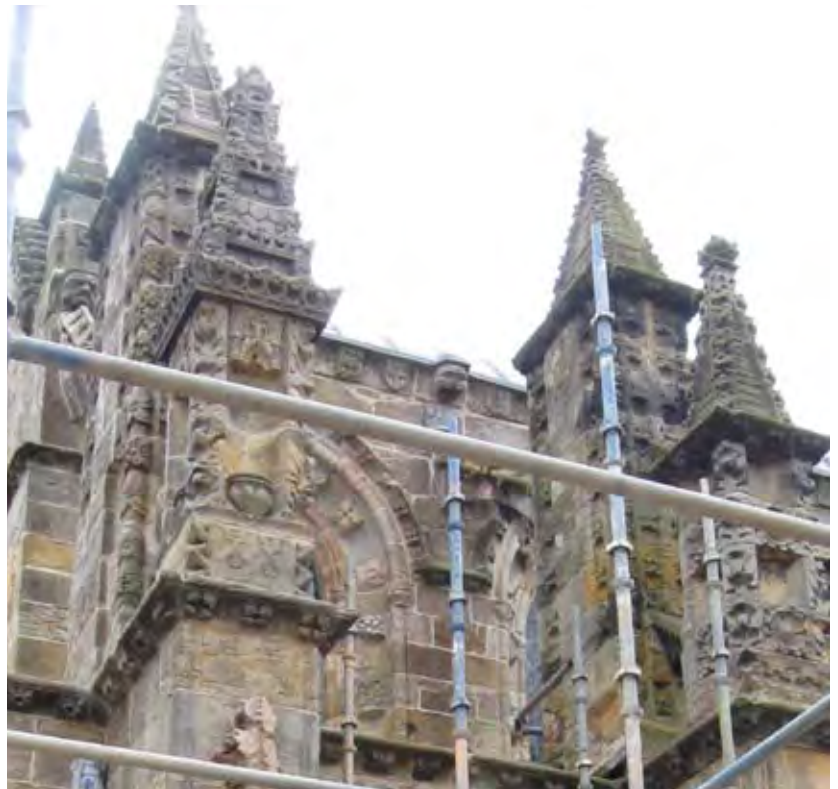
Figure 2.35 North facade with de-soiled and laser treated pinnacles at left and untreated pinnacles at right. July 2011.
