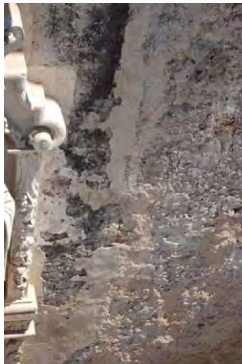
Figure 3.19 Exposed rubble limestone wall adjacent to central carved facade that originally would have been covered in a protective lime render but is now vulnerable to water infiltration.
