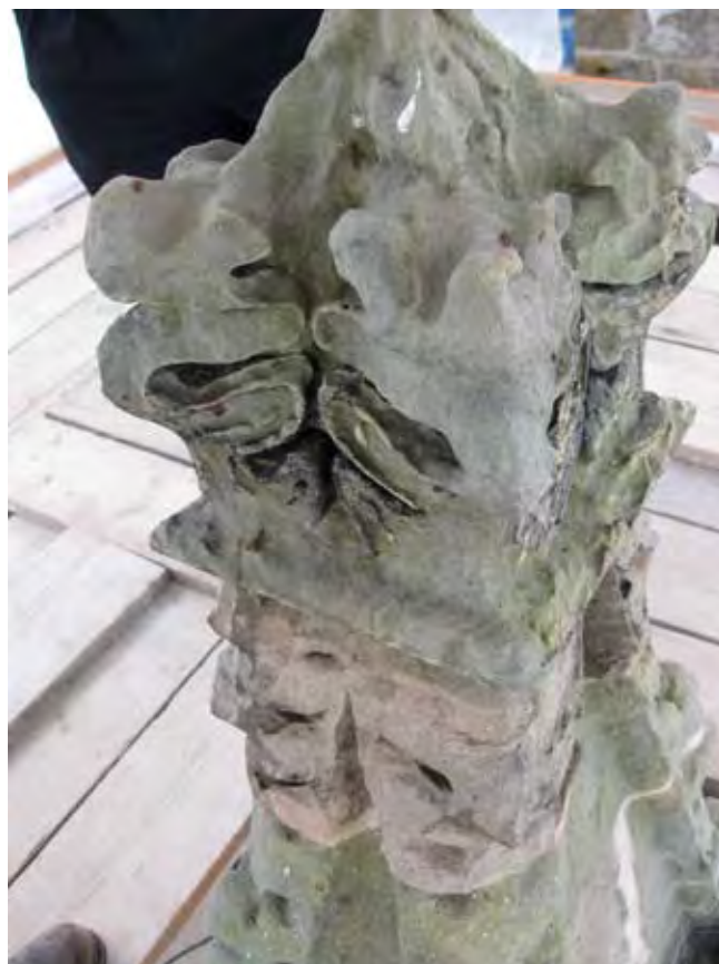
Figure 2.31 Pinnacle at bay S5 after de-soiling and laser treatment and re-pointing of mortar joints, June 2011.
