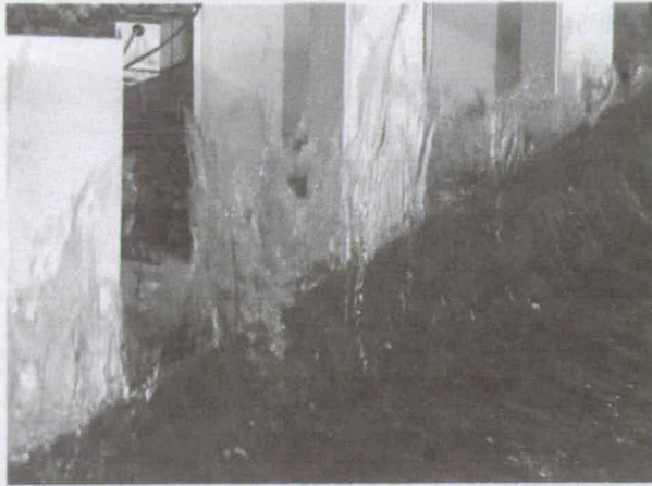
Figure 21: Easily detectable overtopping event (1st highlighted spike, Figure 20)
